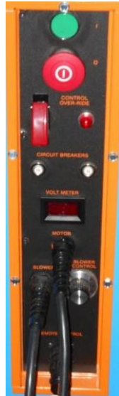
Figure 4 (9218 electrical panel shown)
